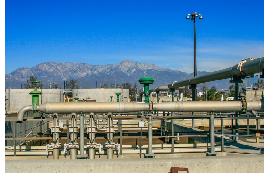
IEUA Regional Water Recycling Plant No. 1 Pipelines
