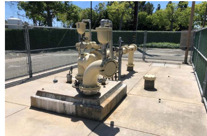
Aquifer Replenishing Wells
